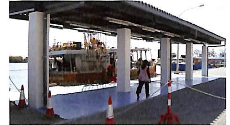
Fish landing and ice restocking quay at Providence fishing port under the Project for Construction of Artisanal Fisheries Facilities in Mahe Island, Seychelles.
